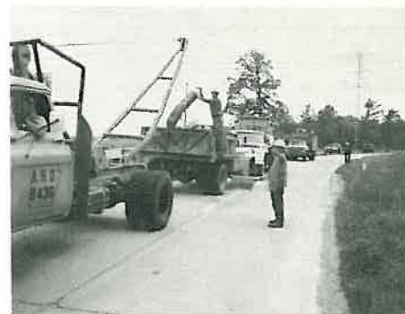
The Monroe County crew pulling old concrete posts to replace them with steel reflectorized posts on Hwy. 1 near the White River Refuge. The truck driver is Lloyd Foster, James Quinn is the flagman and Jerry Morris is loading. That's Ross in the background walking along the edge of the pavement.
